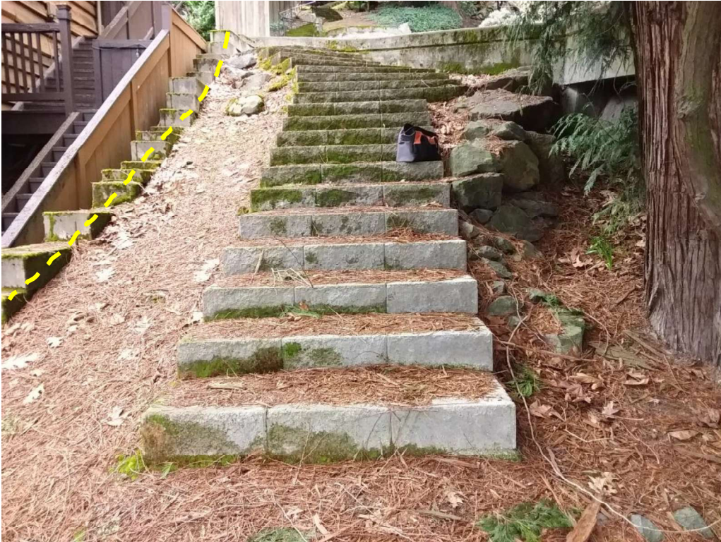
Figure 7. Looking east at the stairs leading up on the north side of the #2 cedar. Note the retaining wall on the left (north) side of the image).
