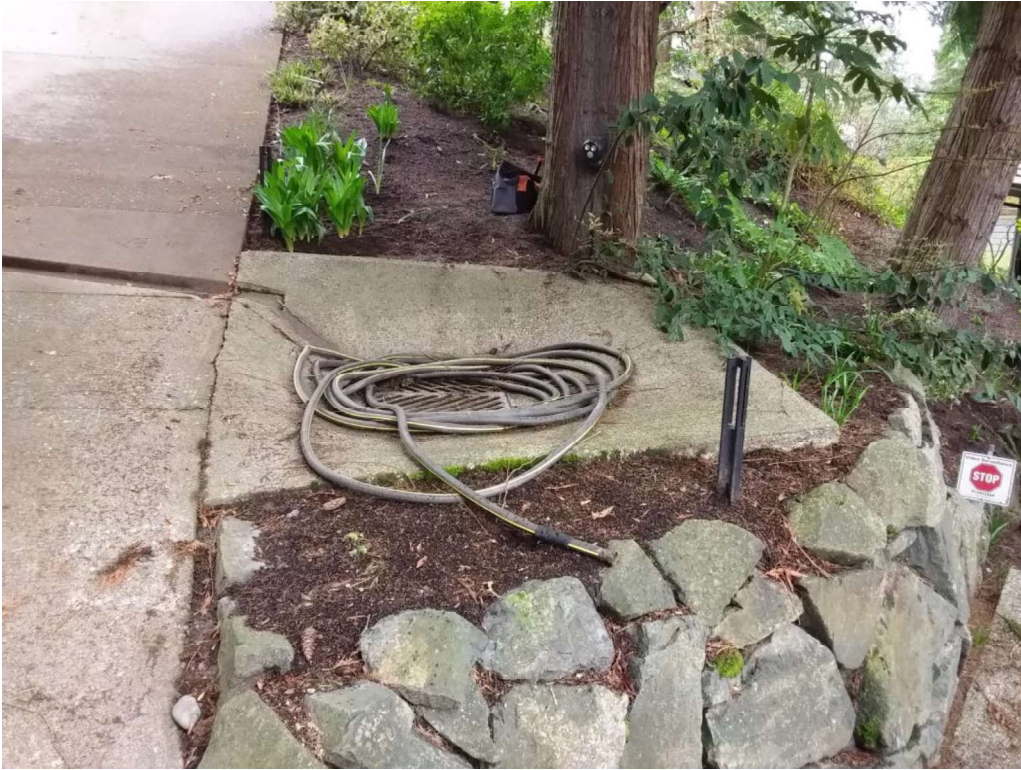
Figure 11. Looking south at the storm drain plate at the base of the #4 cedar. Note proximity of the driveway and stone wall.
