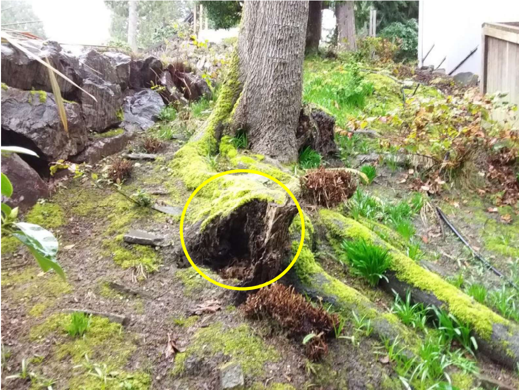
Figure 21. Looking east at the base of the #17 maple from a bit further back. Note the advanced decay in the main structural root.
